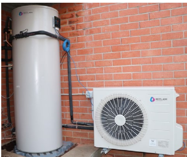
Figure 7: A photo of installed hot water system with proper insulation of pipelines.
