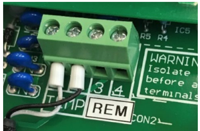
Figure 22: Storage tank terminals 1&2 on block 2 (CON2).
