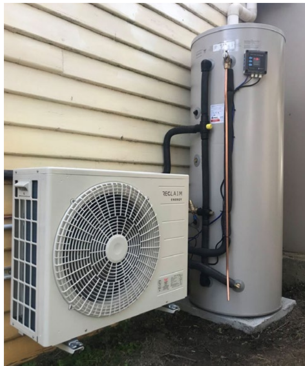
Figure 19: A photo of an installed controller on the tank.
