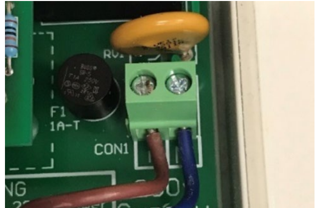
Figure 20: Prewired power cable on terminal block 1 (CON1).
