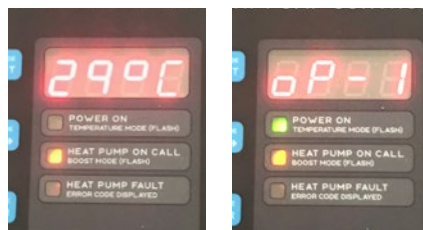
Figure 34: Sample display of controller: tank temperature (left) and active option (right).
